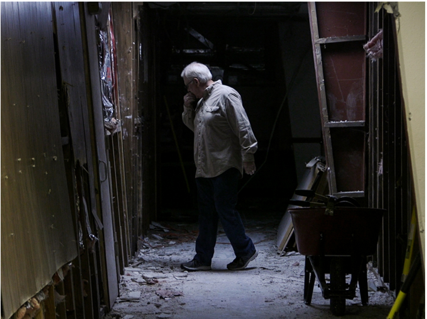
Pastor Charles Stoker looks over damage to Hi-Way Tabernacle Assembly of God Church after Hurricane Harvey in Cleveland, Texas, north of Houston. (Courtesy of Becket Law Firm)
