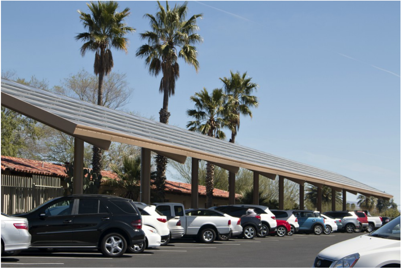
Solar panels reside on a parking canopy at the Carmelite residence near Salpointe High School in Tucson, Arizona. (CNS/Catholic Outlook/Michael Brown)
