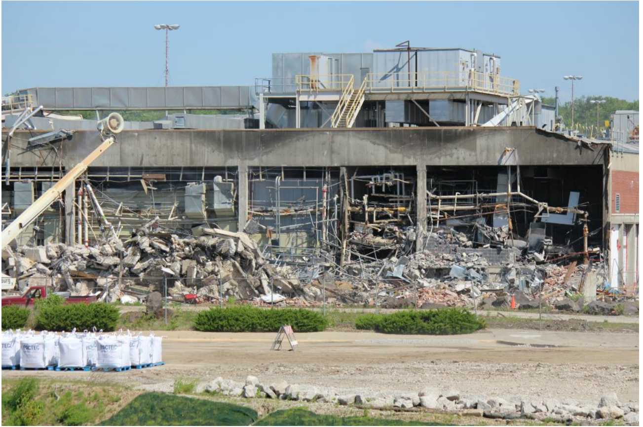
The Kansas City Plant, pictured May 16, 2019, is under demolition by a private developer. (NCR photo/Toni-Ann Ortiz)
