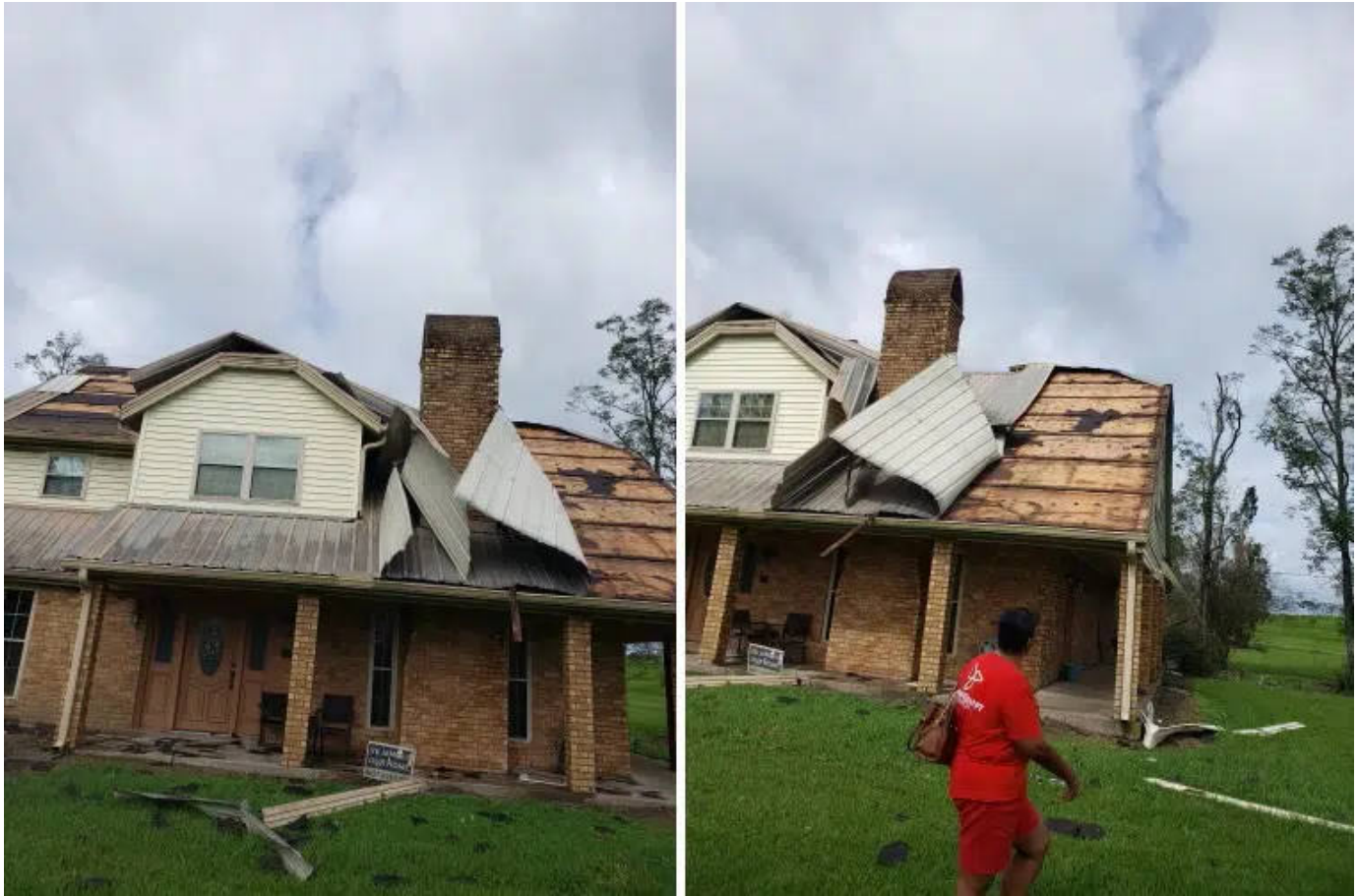
Sharon Lavigne inspects her storm-damaged home in St. James Parish, Louisiana, on Monday, Aug. 30, 2021. (DeSmog/Photos courtesy of RISE St. James)
