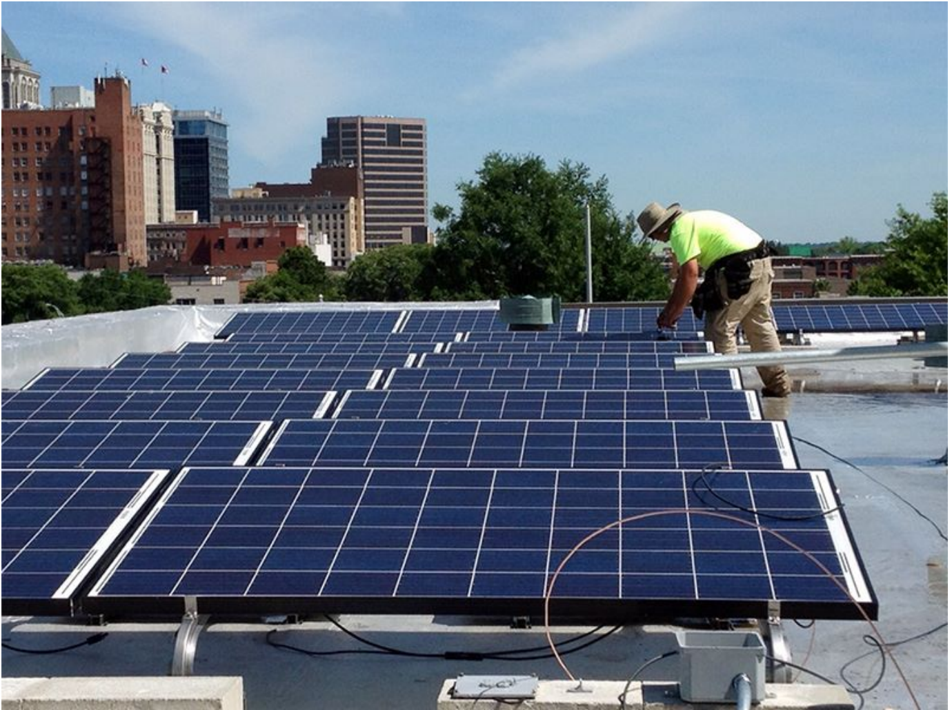
Solar panels are installed on the roof of Faith Community Church in Greensboro, N.C., in May 2015. (Courtesy of NC WARN)
